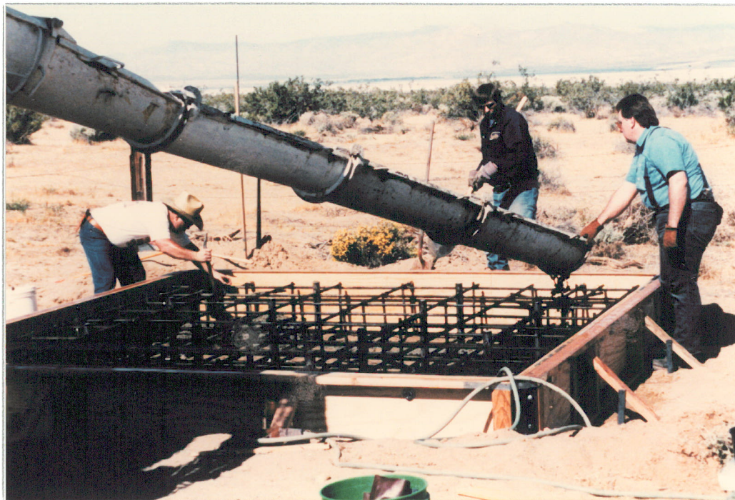
Photo 4 - Chip Basset (left), George Garboden, and Mike Gotlieb (right) start the pour of 10 yards of concrete during the construction of the new 10,000 pound thrust test stand.
