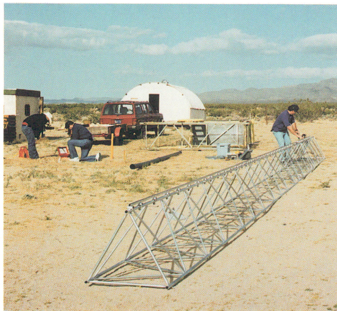
The sixty foot tower being assembled on the ground for its first use in May of 1995.
